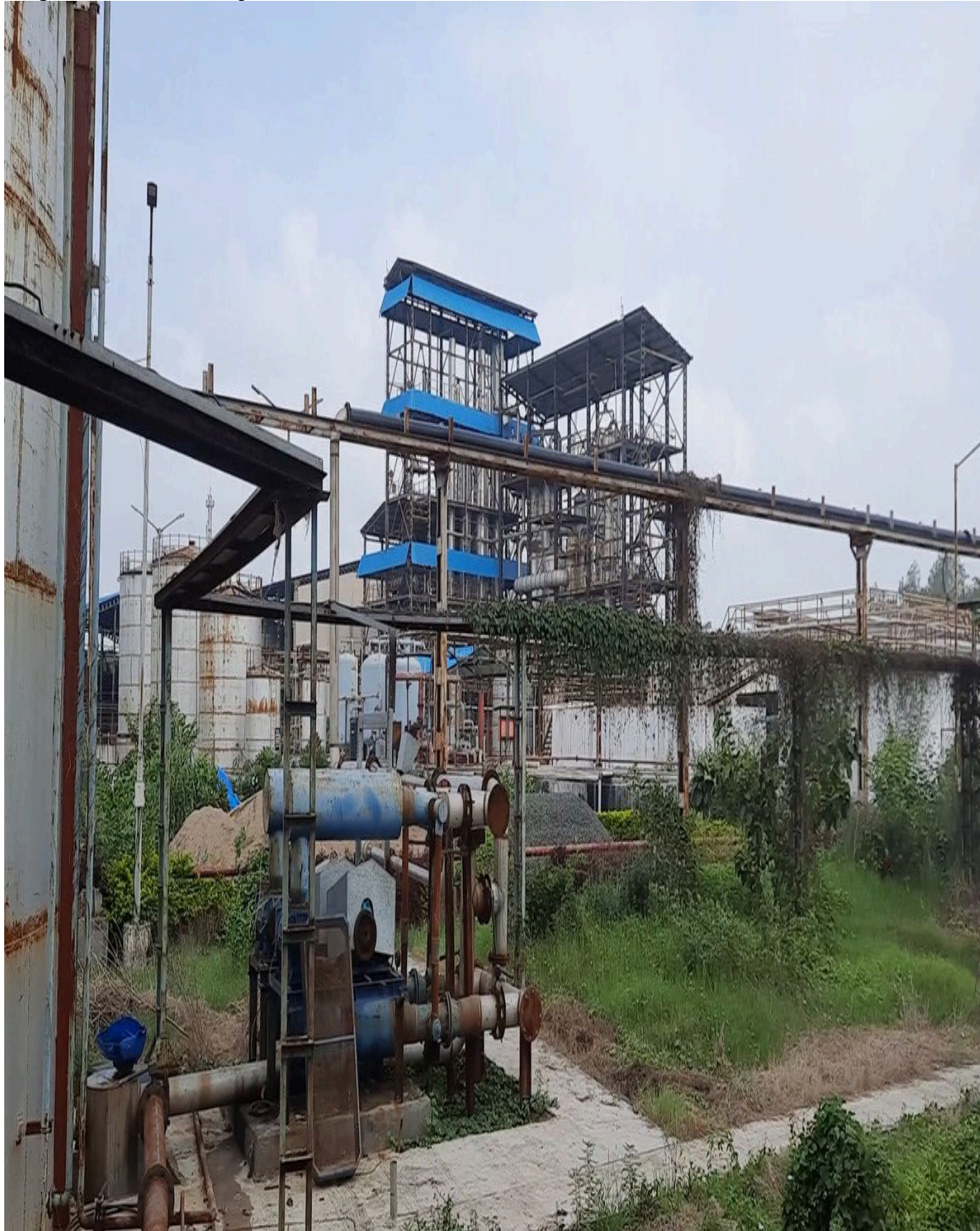
Biogas Holder Blower Pipeline to Boiler:
