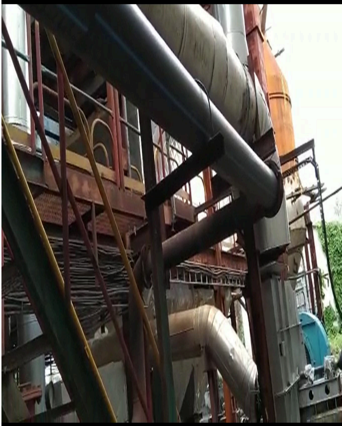
Biogas Pipeline Near Boiler
