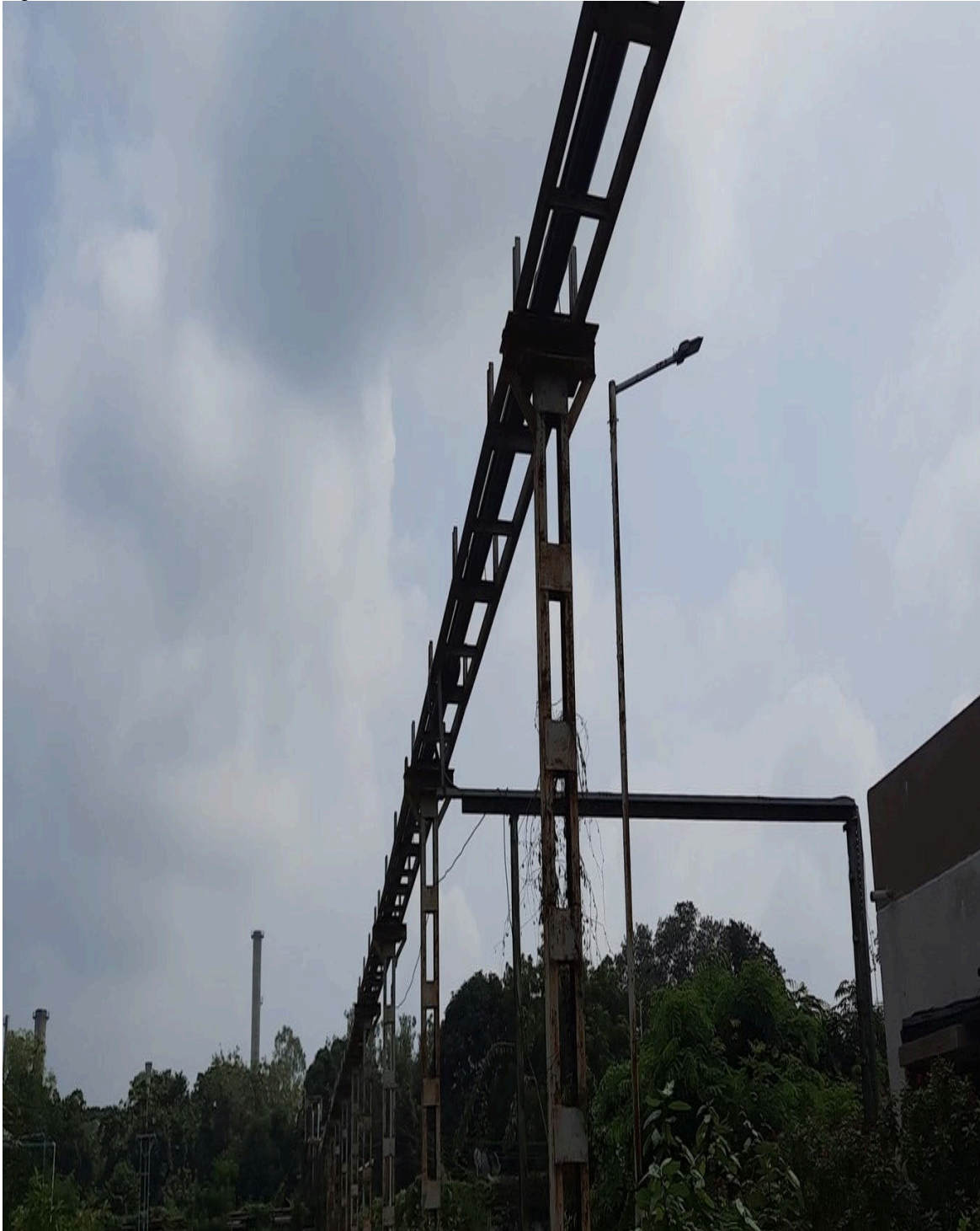
Pipeline to Boiler:
